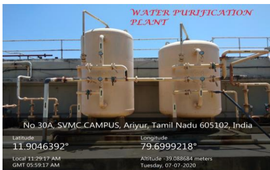
WATER PURIFICATION PLANT
